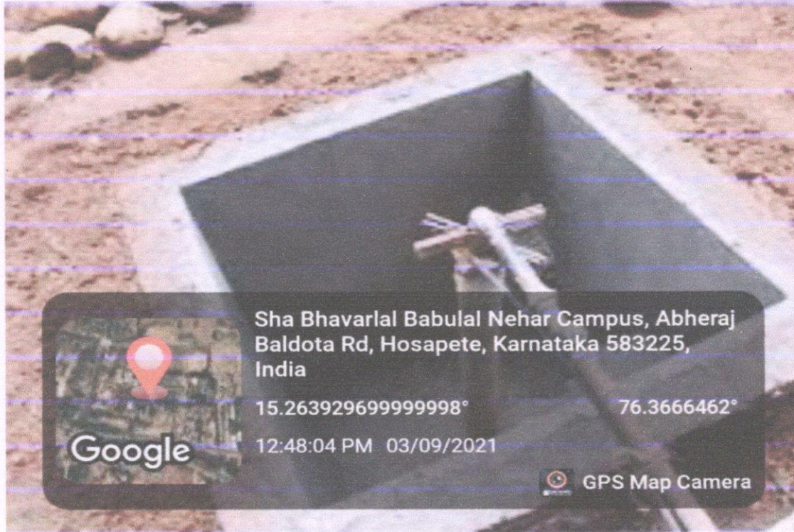
Bore well recharge arrangement
