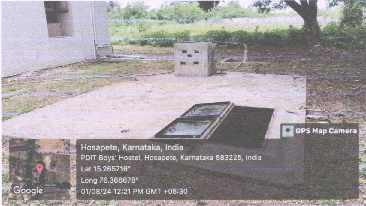
Rain water harvesting in boys hostel.
