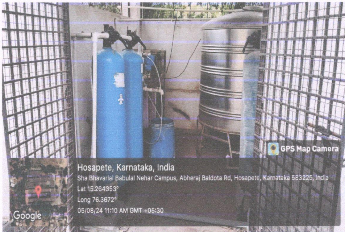
RO water filter unit
